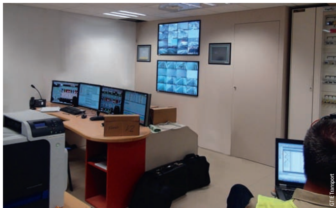
Photo 2 PC secours en tête Saône du tunnel de la Croix Rouse Emergency control centres at Saône head of Croix-Rousse tunnel
