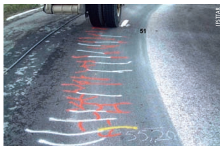
Photo 3 Fissuration de surface observée sur la structure 3 Surface cracking observed on structure 3
