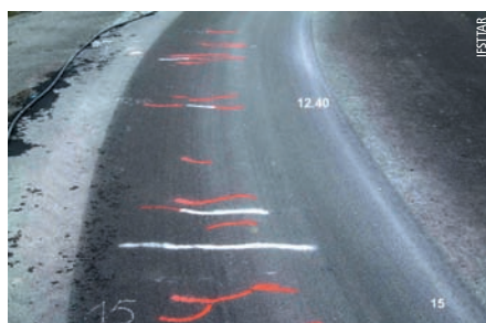
Photo 1 Fissuration de surface observée sur la structure 1 Surface cracking observed on structure 1
