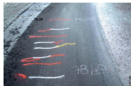
Photo 4 Fissuration de surface observée sur la structure 4 Surface cracking observed on structure 4
