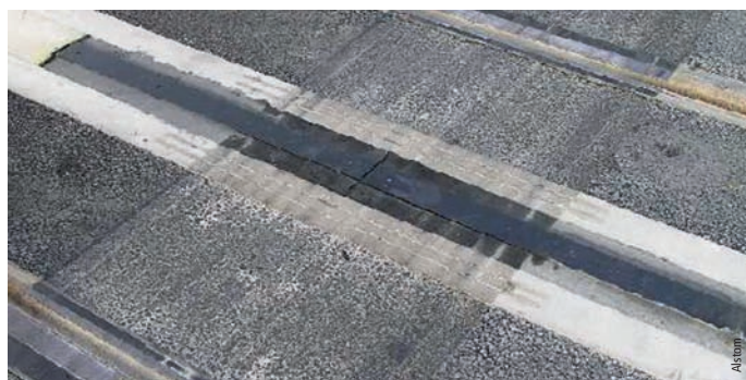
Photo 4 Poutre béton rail isolant revêtement BB percolé orniéré Concrete beam, insulating rail, percolated and rutted asphalt surfacing
