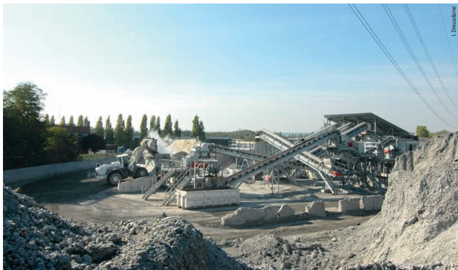
Installation SPL de maturation et d'élaboration de Saint-Ouen-l'Aumône SPL maturing and manufacturing Installation of Saint-Ouen-l'Aumône
