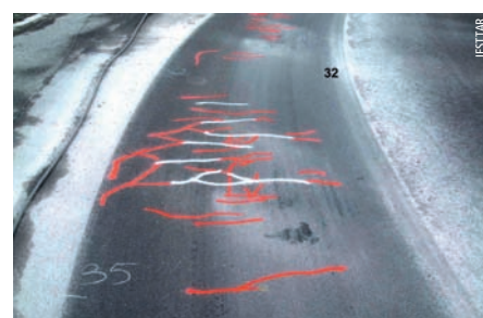
Photo 2 Fissuration de surface observée sur la structure 2 Surface cracking observed on structure 2
