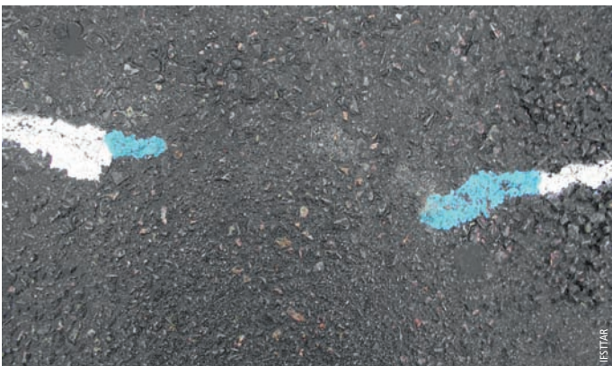
Photo 10 Evolution de la fissure à 426 000 passages Evolution of crack after 426,000 passages
