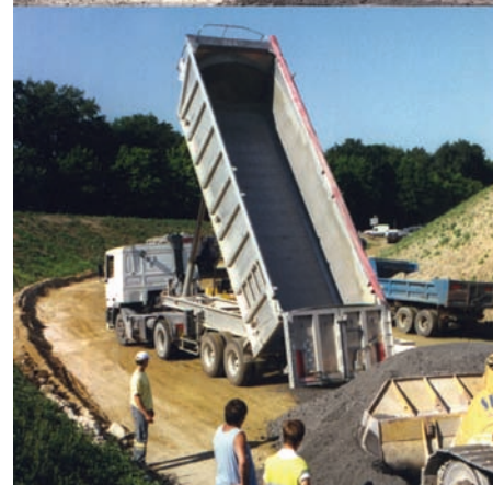
Chantier Scorcim sur RN, charte innovation Sétra Scorcim worksite on national highway in connection with Setra innovation charter
